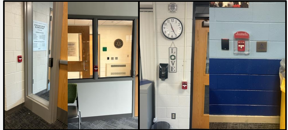
Stadium Drive and Webber Elementary Pull Station Relocation Finalization
