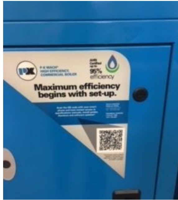
High School, Scripps and Orion Oaks- New P-K Mach 95% Efficiency Boilers
