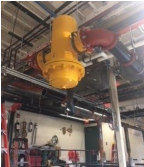
Scripps Middle School- Air and Dirt Separator.
