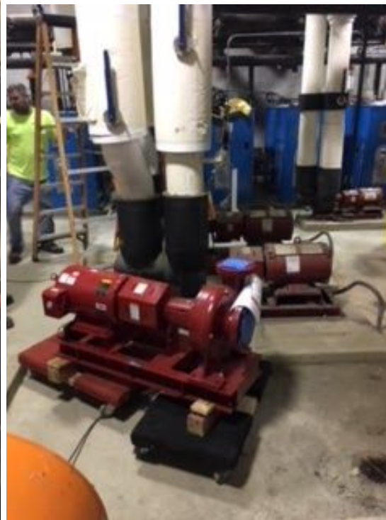
High School- New Secondary Loop Pump
