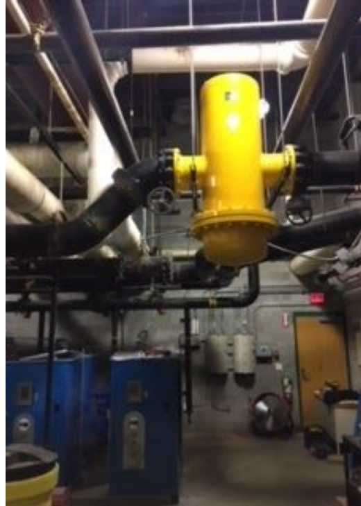
High School - Air and Dirt Separator installed
